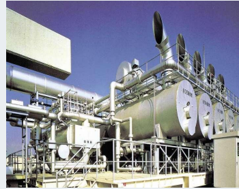
<Environmental protection equipment>
