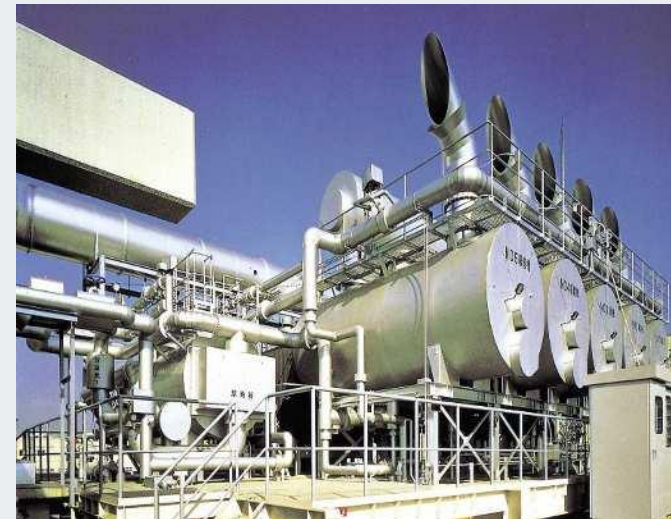
<Environmental protection equipment>
